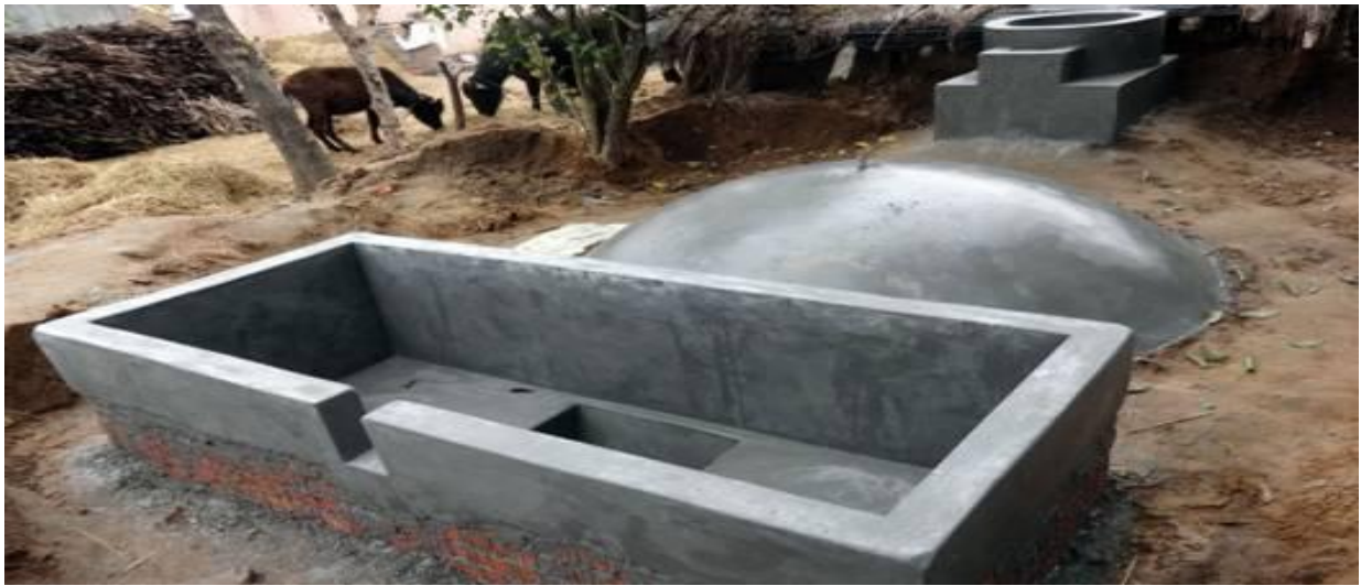
A view of installed biogas plant.
