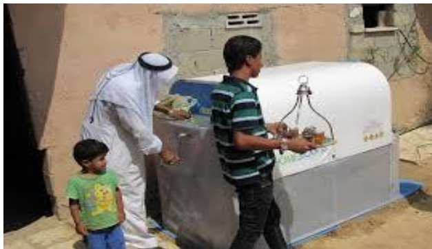
The HomeBioGas in local area in Israel
